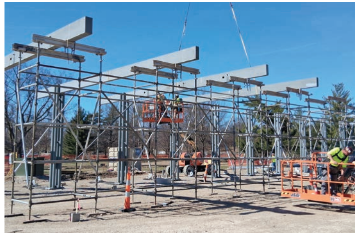
Vertical columns with cantilevered beams will form the shade structure west of the rink.
