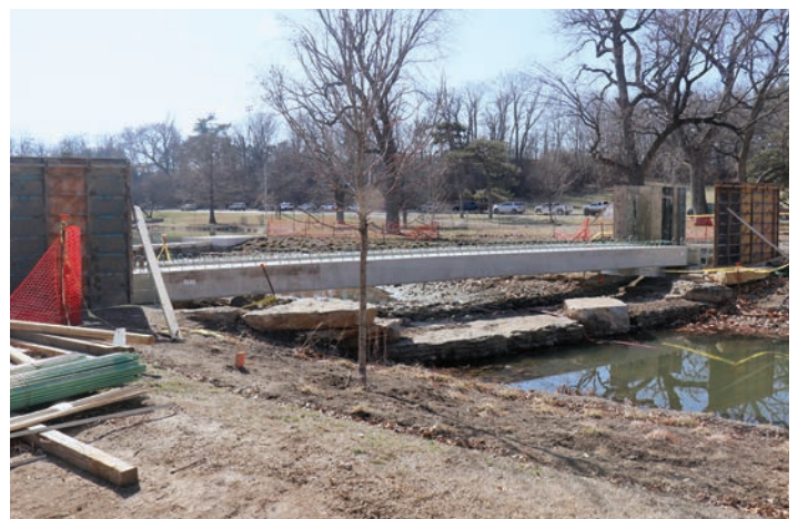
Girders for the new pedestrian bridge over the Taylor Kindle River west of the Glade site.
